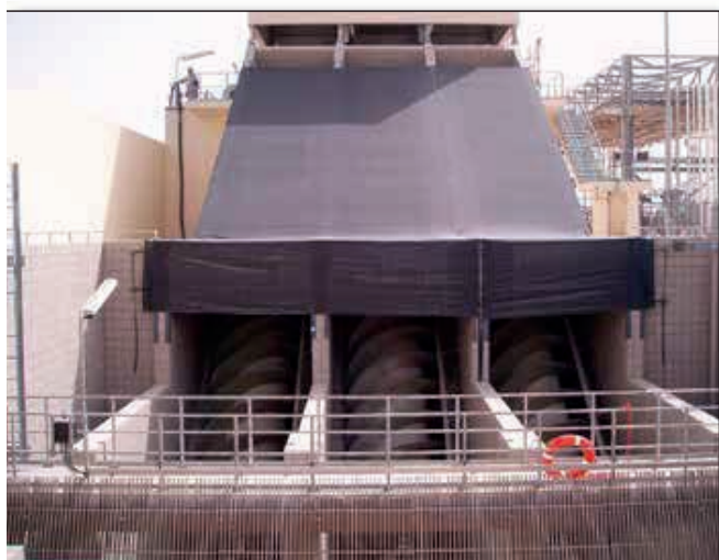
Ras Laffan, Qatar
